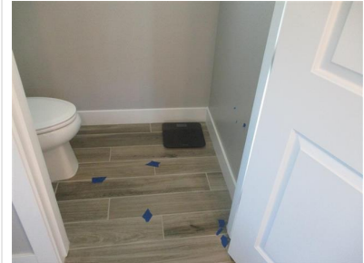
7.1 Item 5 (Picture) master toilet closet
